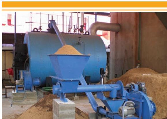
Paddy husk heated boiler - Katana: funded under e-friends scheme
